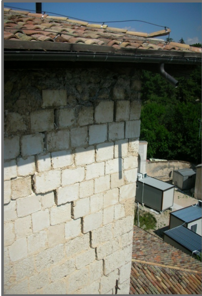
Damage C on the apse
